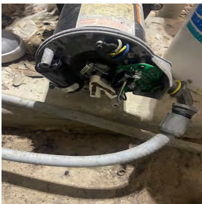
Bad Filter Pump Motor
